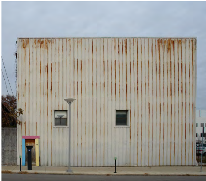
South Facade, Metal, Glazing, Plywood Board Up
